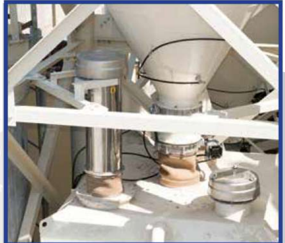
Filters and Safety Valves
