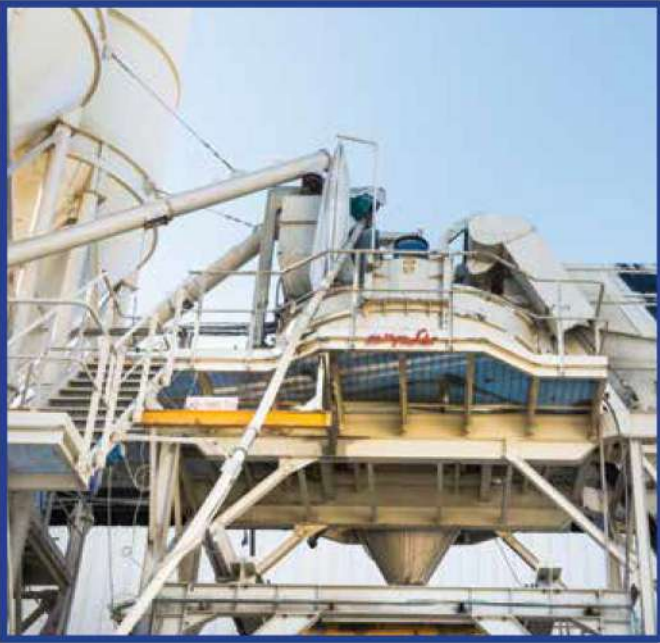
Mixers for wet plant
